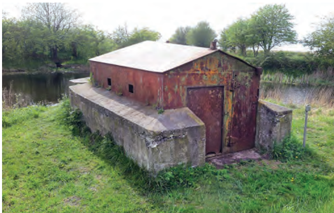
Unusual iron caponier protecting the moat of Kongelunds Fort which can still be seen in water beyond it
